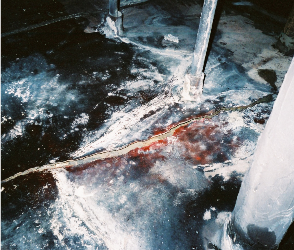
Fiberglass High Temp Damage
