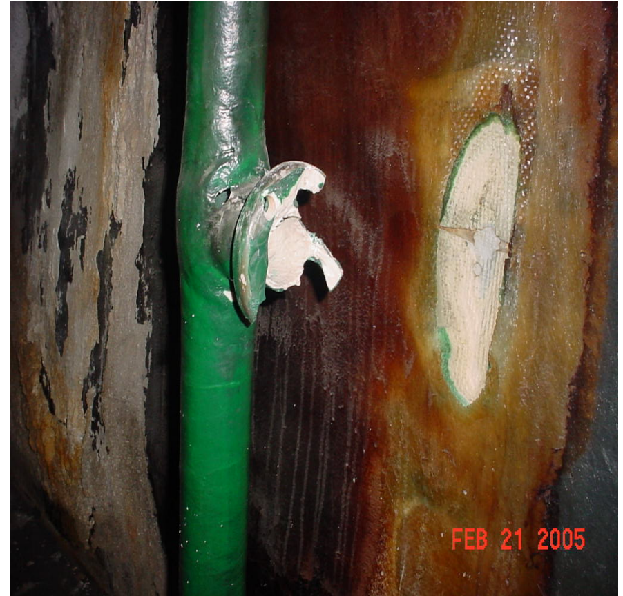
Fiberglass Abrasion Damage
